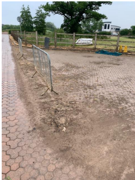
Surface mud on thrid exit of roundabout
